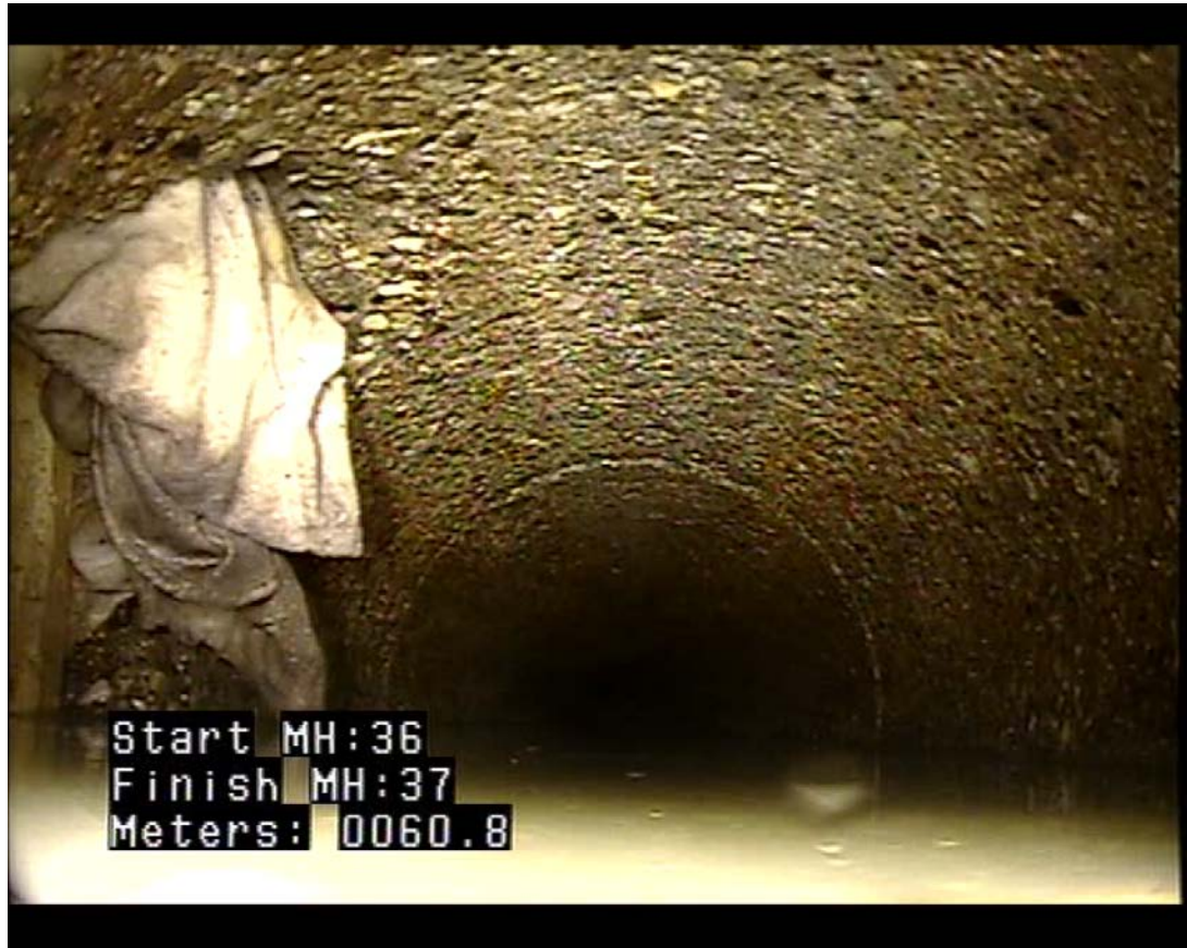
Photo 5.2: Rag Wrapped around Service Pipe in Highwood Drive (SP 125)
