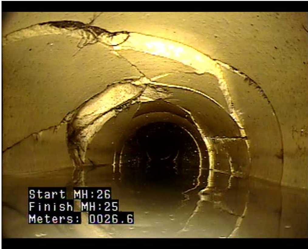
Photo 5.1: Severe Cracking and Fractures near Service Connection in Twin Cities Drive (SP 139)
